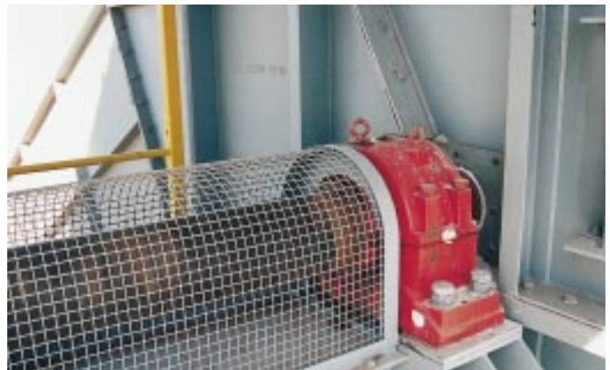
Ventilator drive unit
