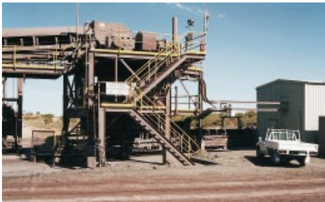
Conveyor plant drive unit
